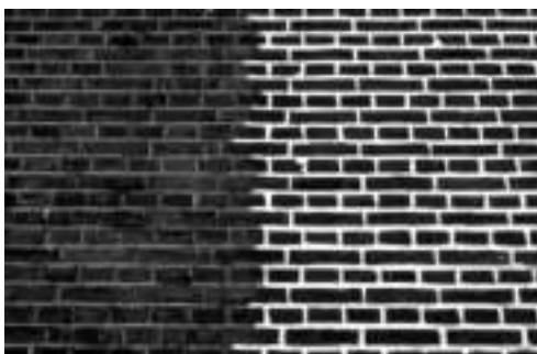
Figure 1 : The aspect of the façade changes completely, when colour or even shape of the pointing changes.
