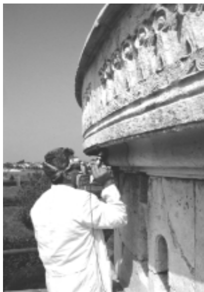
Figure 6 : The Mausoleum of Teodorico under restoration. The laser can be noted on the left at ground level. The cleaning operation on the scaffolding is carried on by means of the optical fibre handpiece.
