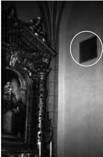
Figure 2 : Outlet grid of a hot air heating system. A violent airflow of hot air is ejected in proximity of wooden altar and canvas painting.
