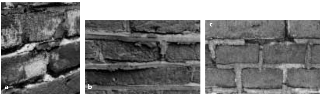
Figure 2a, b, c : Look alike damage : push out of pointing due to different processes (salt crystallisation, swelling pointing mortar, frost action to bedding mortar).
